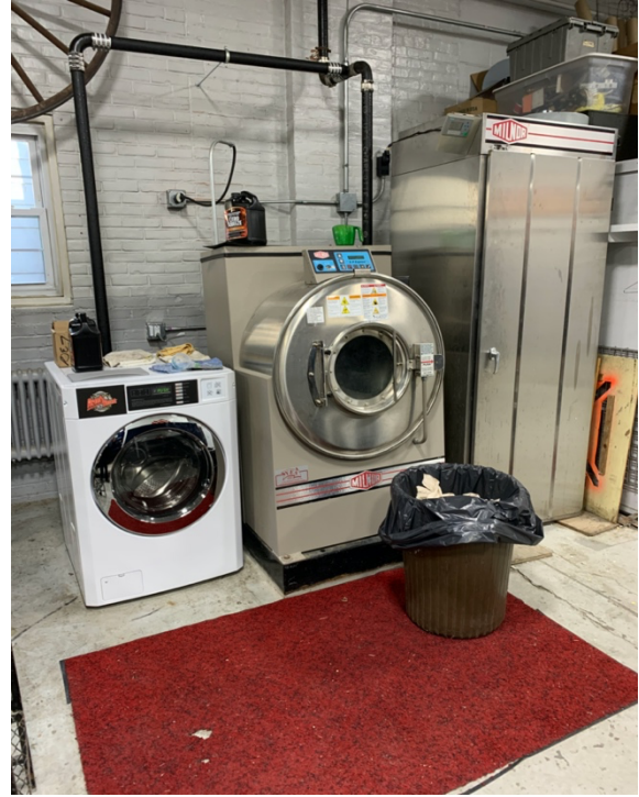
Figure V-11 Outdated Plumbing and Fixtures
